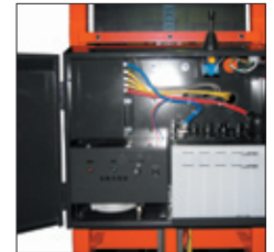
Inside unit box
